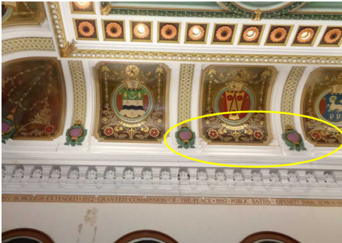
Initial Dry Rot Outbreak Below the Lancashire Panel
